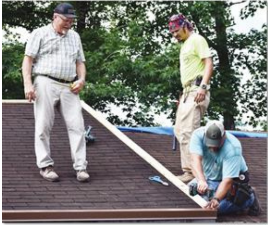
Workers from Bethany United Methodist Church in Summerville, S.C. work on the roof of a home at 912 Turner St. Monday morning. The mission group, part of the United Methodist Committee on Relief, is to soon this week working on the home to repair it after storm-damaged damage to it in December 2015.
